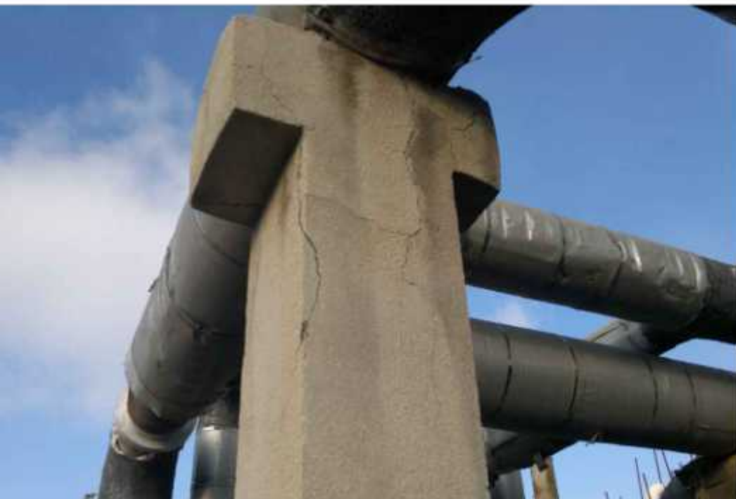
Project title: Renewal and rehabilitation of the foundations of the Kharg factories Employer: Iran Offshore Oil Co. Location: Khark Island
