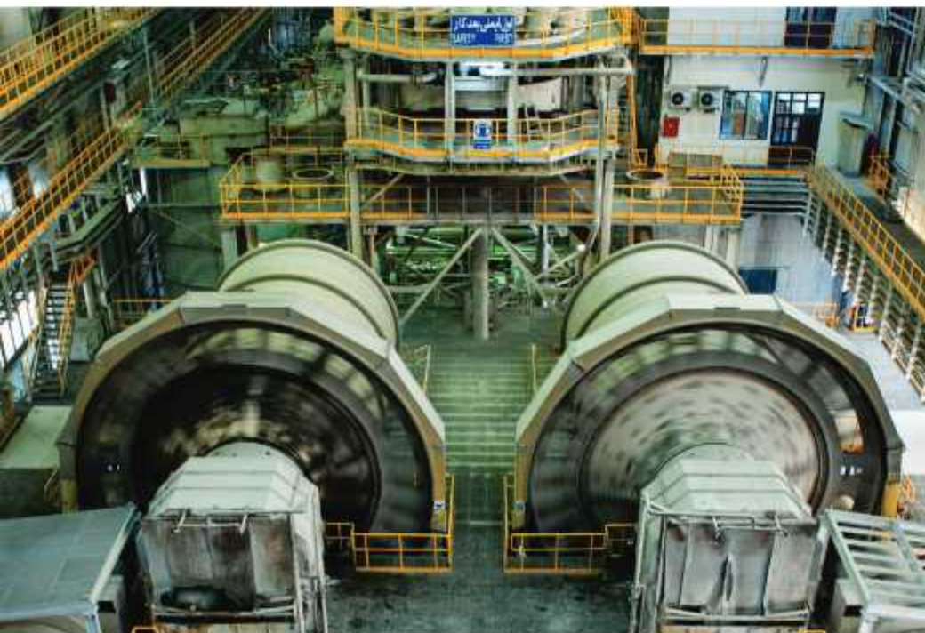
Project title: SUNGUN copper condensing plant Employer: National Copper Industry of Iran Location: Eastern AZERBAIJAN, VARZAGHAN
